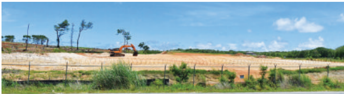
SITE WORK: Work continues to pave way for facilities within Marine Corps Camp Blaz which will host nearly 5,000 Marines who will be relocated from Okinawa. This was seen along Route 3 in Dededo on Sunday. David Castro/The Guam Daily Post
